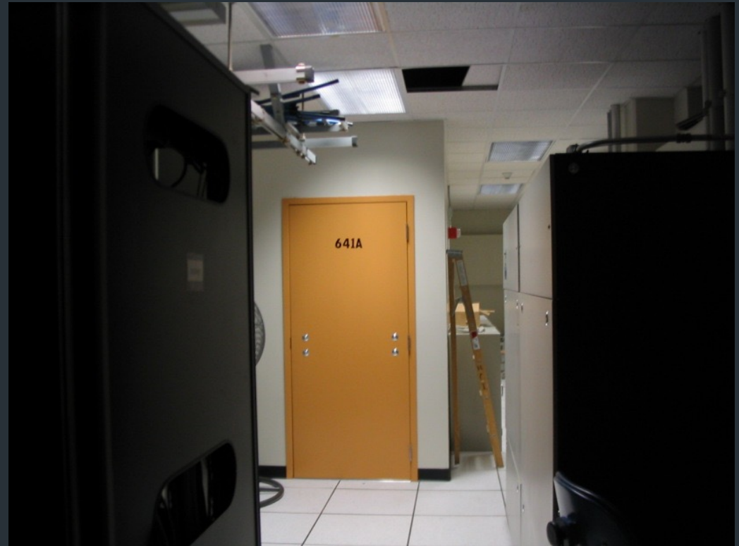
Room 641A: wiretapping room in a datacenter for an Internet backbone...
