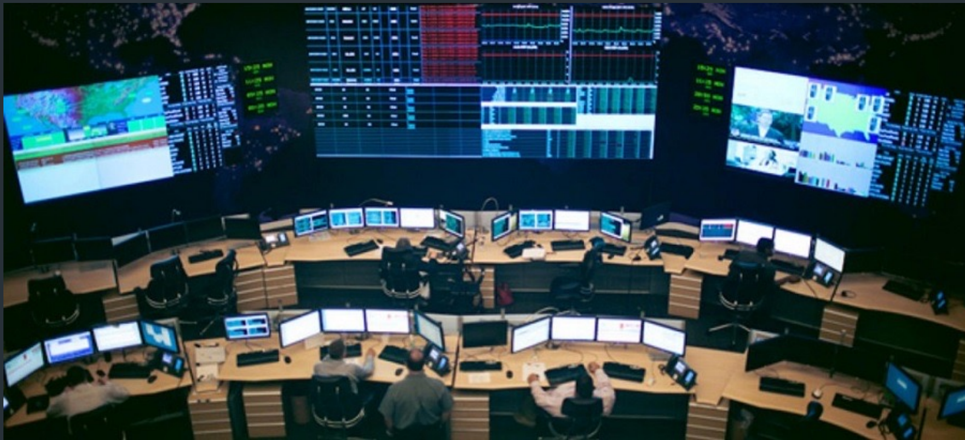
A Network Operations Center (NOC)
