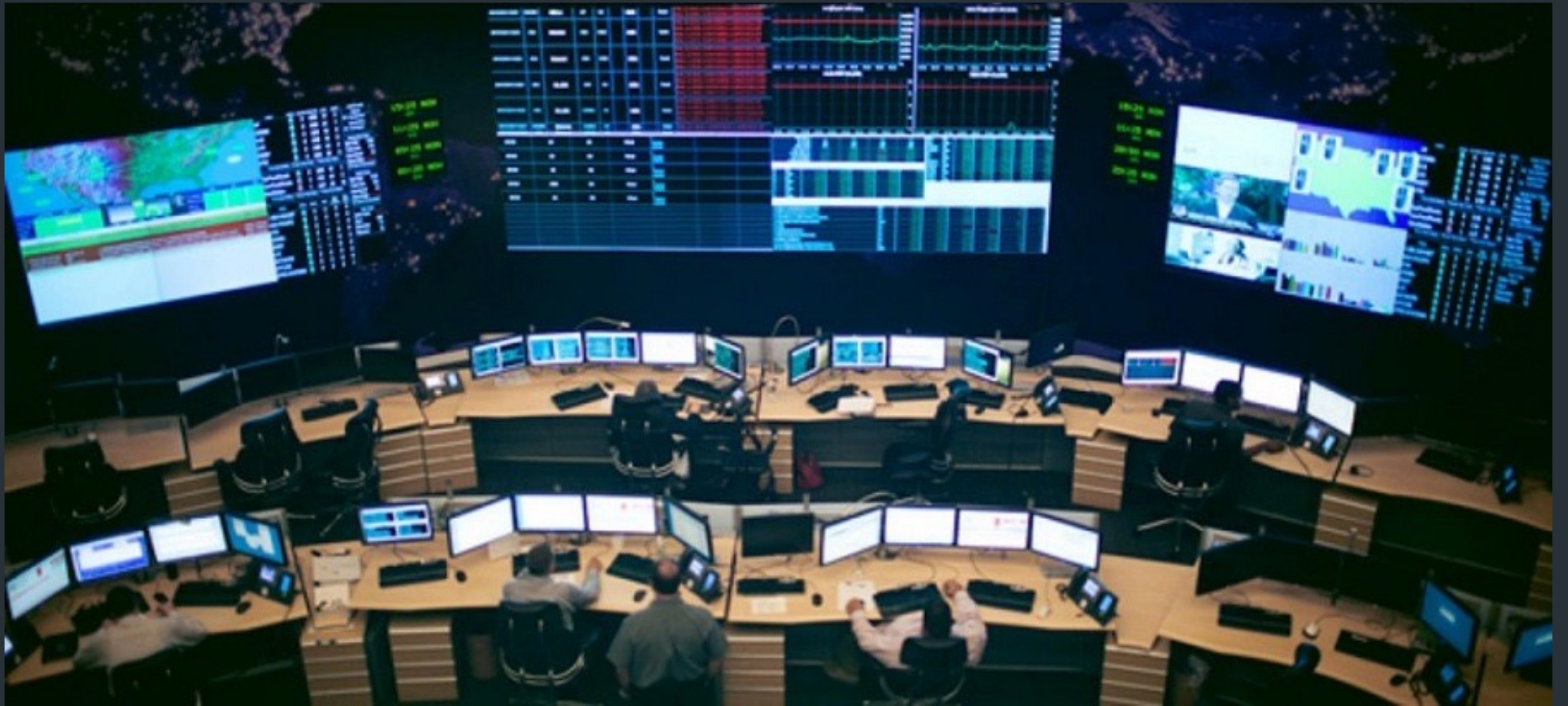
A Network Operations Center (NOC)
