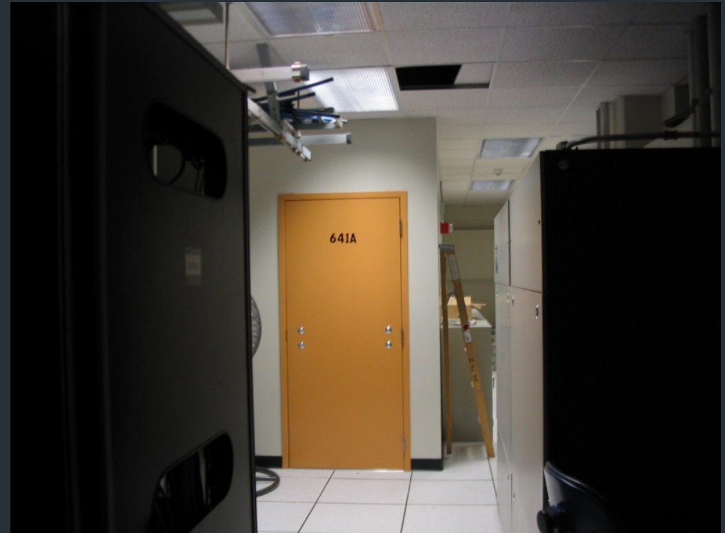
Room 641A: alleged wiretapping room in a datacenter for an Internet backbone...
